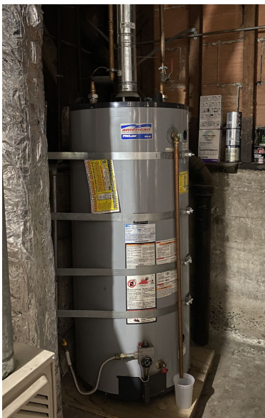
Gas water heater
