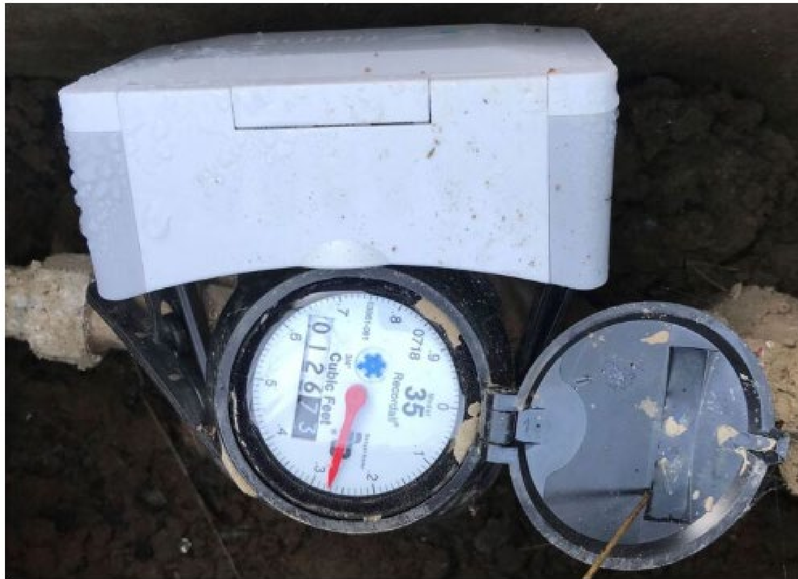
Pictured is a water meter photographed from above with a flowmeter attached to the side.
