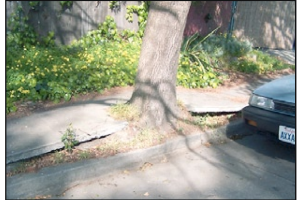
Some Rockridge sidewalks have been dramatically affected by tree roots. Is removal the only option?
