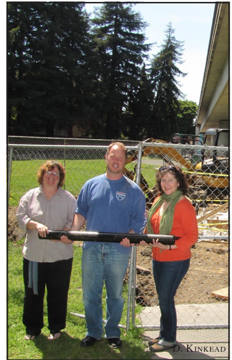
Ronnie Spitzer, left, Mike McDonald and Theresa Nelson at the construction site of the new Frog Park restroom.
