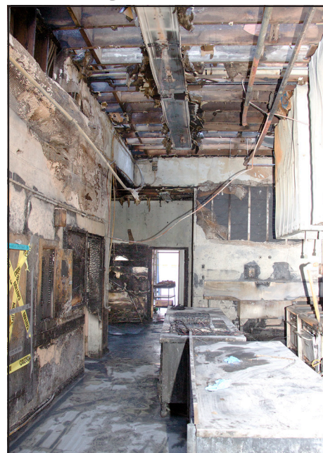
Fire destroyed the Claremont Middle School kitchen and cafeteria in mid-February, 2015. Planning and design for its replacement, along with other campus construction projects, are underway. /D. KINKEAD
