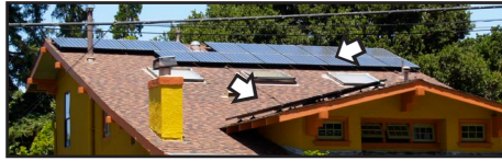
South- and west-facing solar panels installed on a Rockridge Bungalow home. PHOTO: DON KINKEAD
