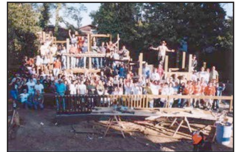
2001: Hardy Park Big Build participants celebrate their playground construction progress. PHOTO: BILL CALDWELL
