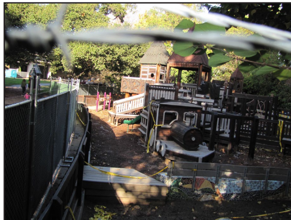
Hardy Park play structures are temporarily fenced off for repairs. PHOTO: D. KINKEAD
