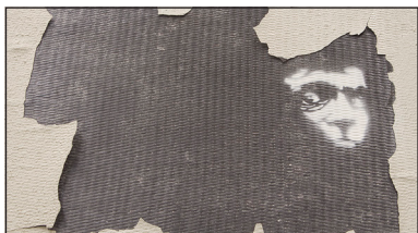
The paint chips flaking from the pillars in the BART parking lot recently revealed a possible cause of the blight lurking beneath the surface. /D. KINKEAD
